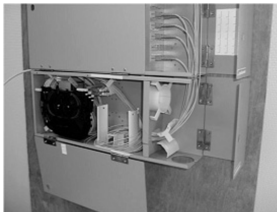
Fig. 7 Optical connection box for the pilot.
